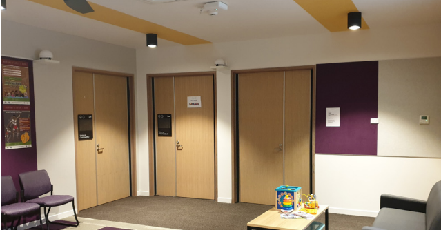
Waiting area with under floor transducers on floating shelves
