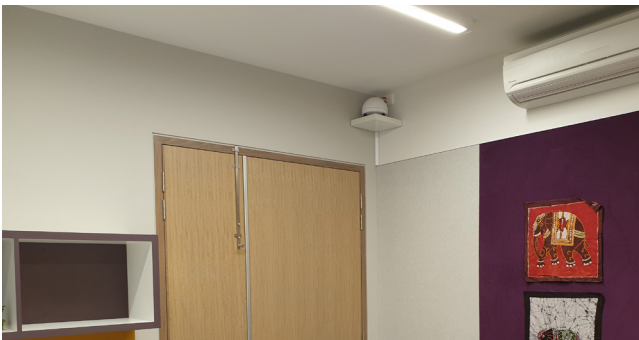
Transducer installed in office on high corner floating shelf
