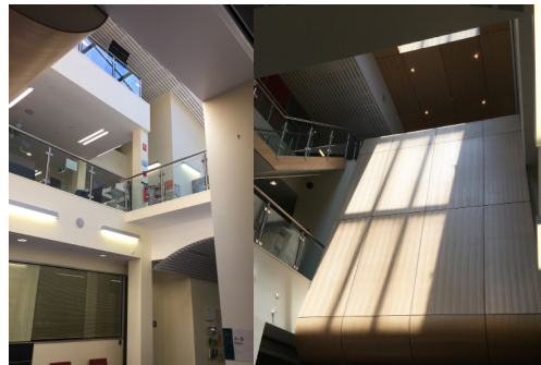
The atrium – noise transfer was exacerbated by the wooden facade
