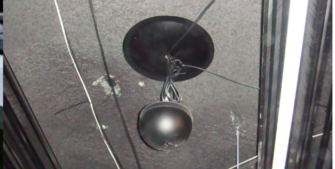
Installed transducer with acoustic disc
