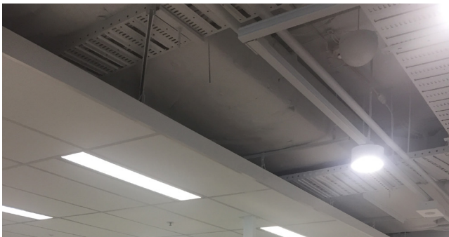
Soundmask transducer in open ceiling area
